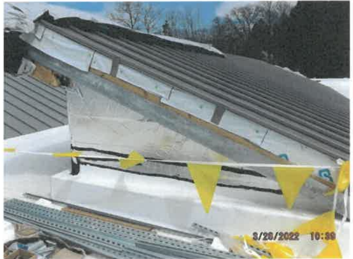
Photo depicts the progress of the metal at sawtooth roofs on the apparatus bay.
