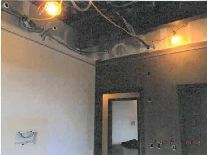
Photo depicts the progress of the third floor finishes—Paint and ceiling grid.
