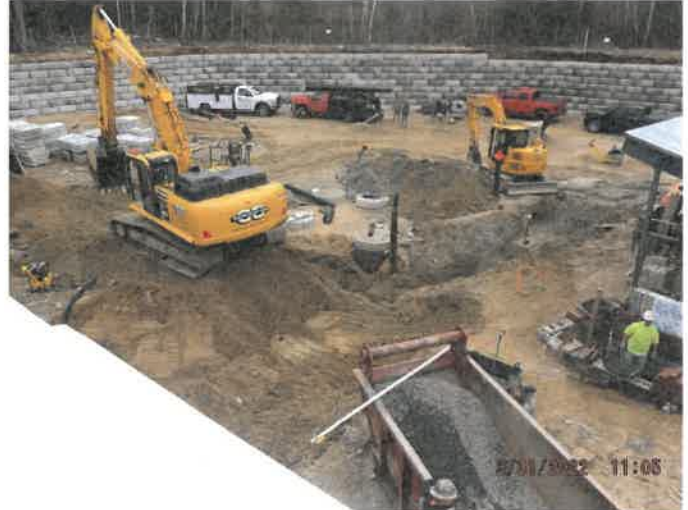
Photo depicts the progress of drainage at the rear of the site.
