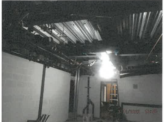
Photo depicts the progress of block-filler in the apparatus support room area.
