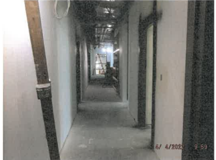
Photo depicts the progress of the Second floor paint and insulated duct.
