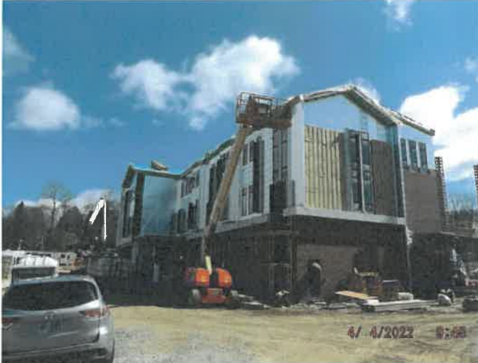
Photo depicts the progress of the AVB, window installation, window trim, brick, and secondary wall framing.
