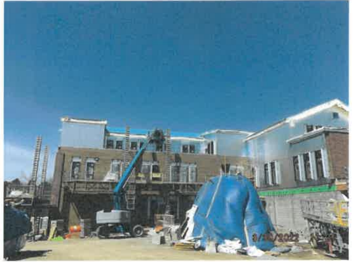
Photo depicts the progress of the AVB, framing, window installation, window trim and brick.
