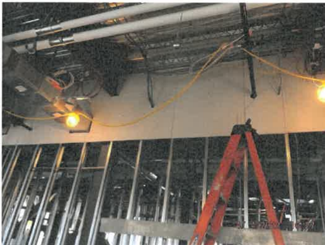
Photo depicts the progress of First floor drywall, insulated plumbing and HVAC piping and sprinkler heads.
