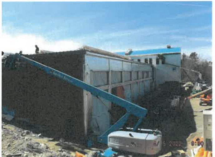
Photo depicts the progress of the AVB at the apparatus bay and metal roof soffit.
