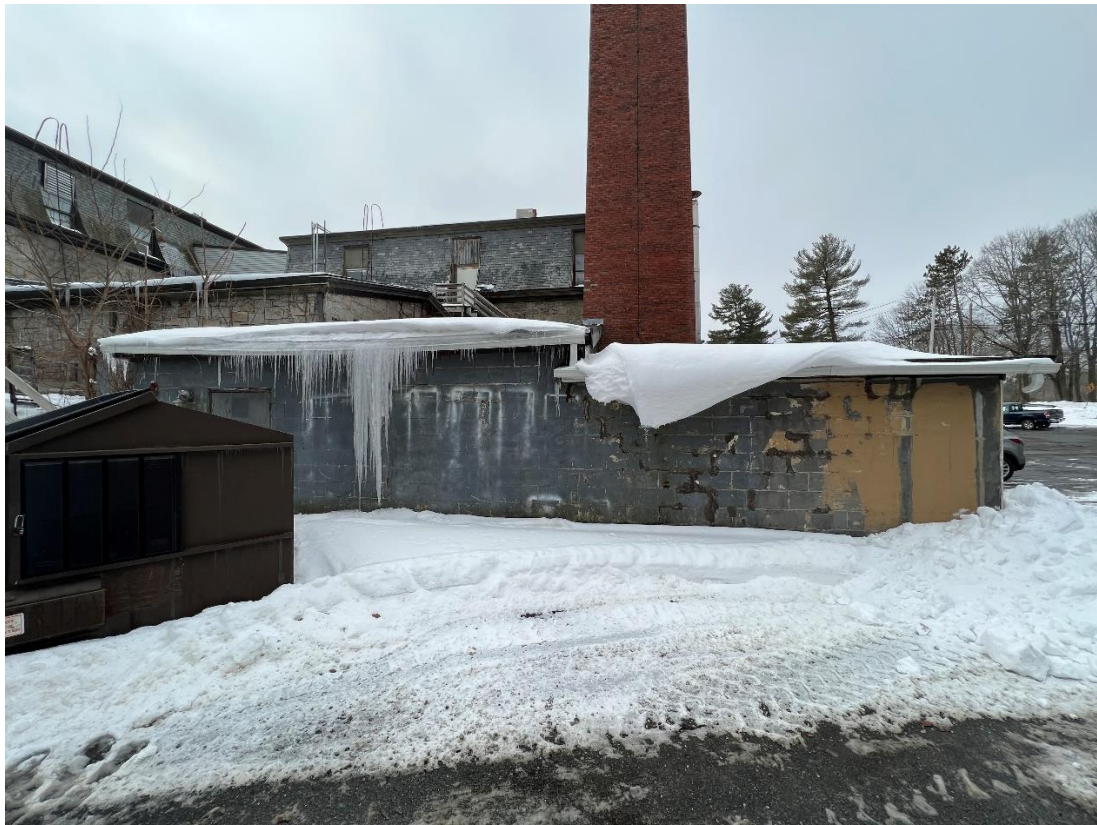
10-20 Main – Bottom photo - one story additions to the rear are to be removed – chimney remains
