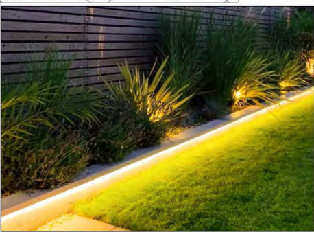
IN-GROUND LED STRIP LIGHTING
