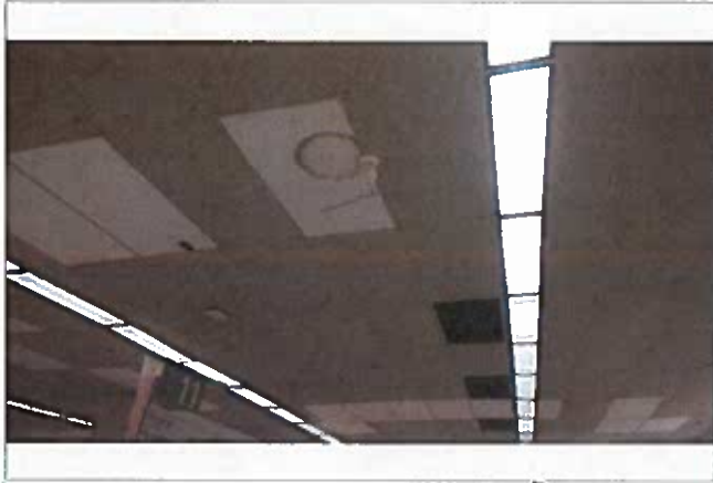
Stained ceiling tile
