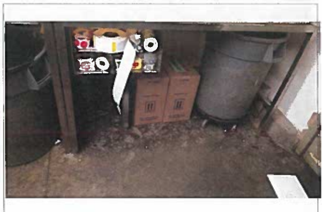
Produce back room floors with debris and soils
