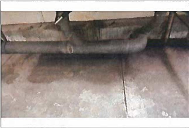
Leaking sink drain.
