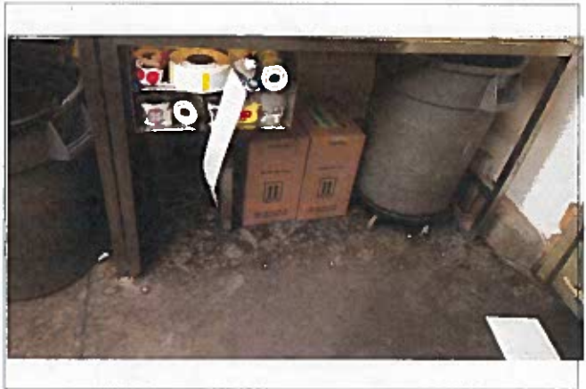
Produce floors need to be resurfaced.
