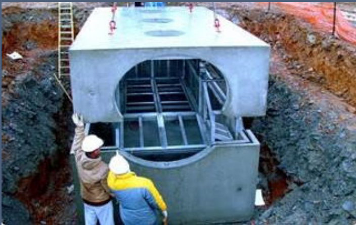
Typical Electrical Vault
