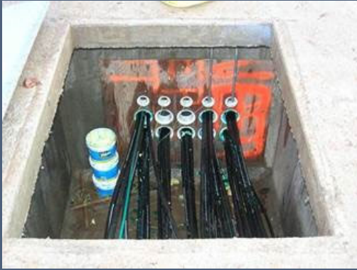
Typical Electrical Vault
