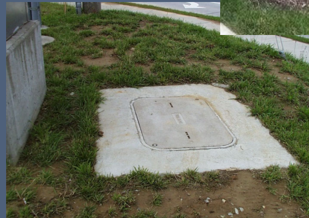
Typical Electrical Pull Box
