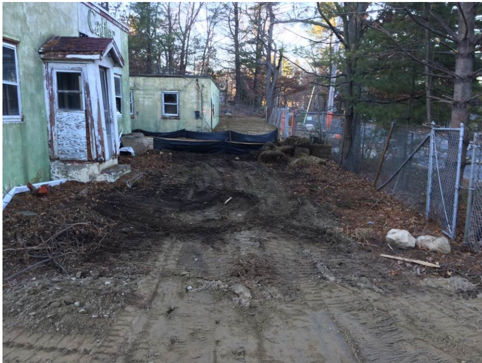
SCENE: View of final site conditions north of the office building. Photograph taken facing northwest.
