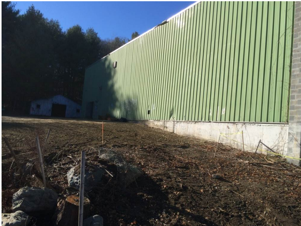
SCENE: View of the area south of manufacturing building following backfilling. Photograph taken facing west.
