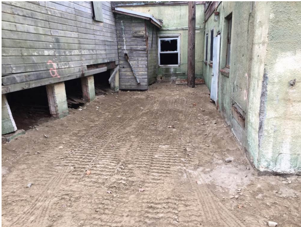
SCENE: View of the indented contaminated soil excavated area along the southeastern side of the lab building following backfilling activities. Photograph taken facing northwest.
