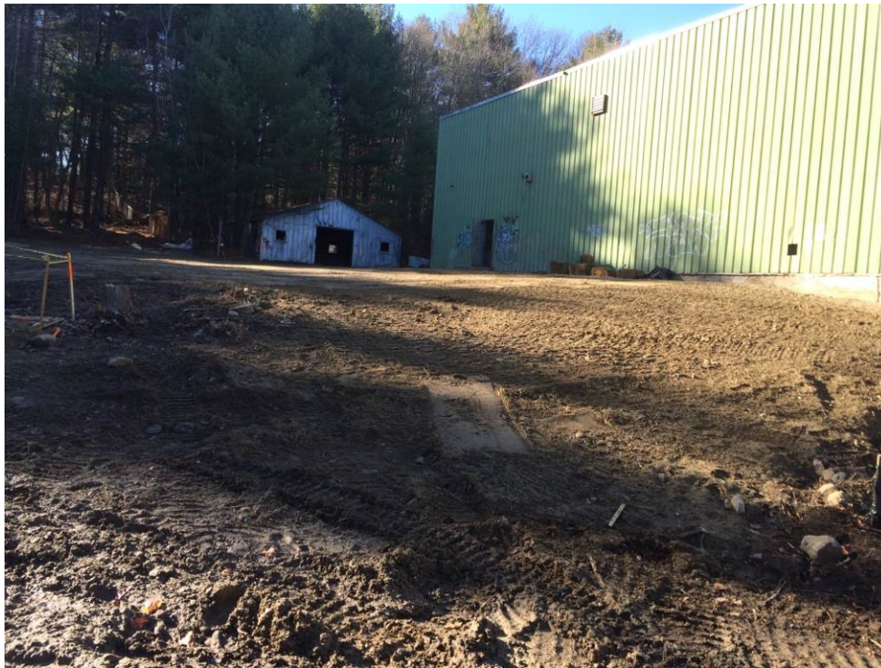
SCENE: View of the area south of manufacturing building following backfilling. Photograph taken facing west.
