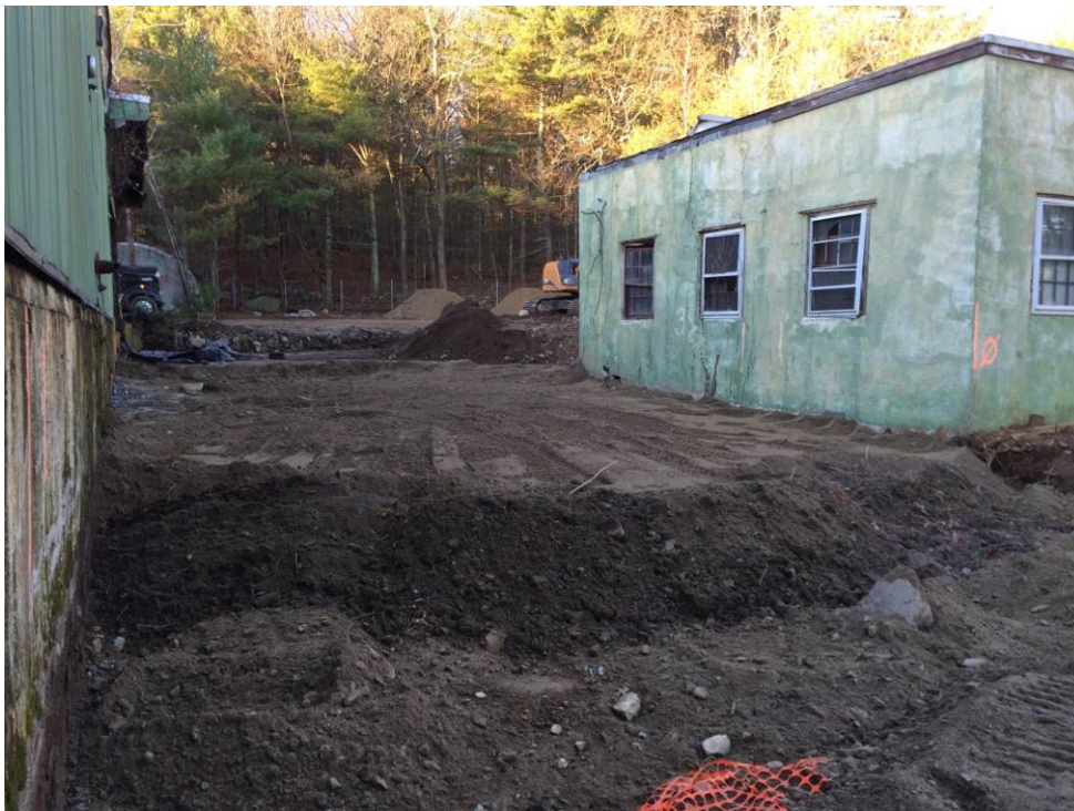
SCENE: View of the area between manufacturing and office buildings during backfilling. Photograph taken facing southwest.
