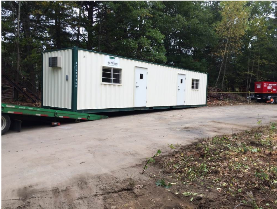
SCENE: View of the office trailer during unloading. Photograph taken facing southeast.
