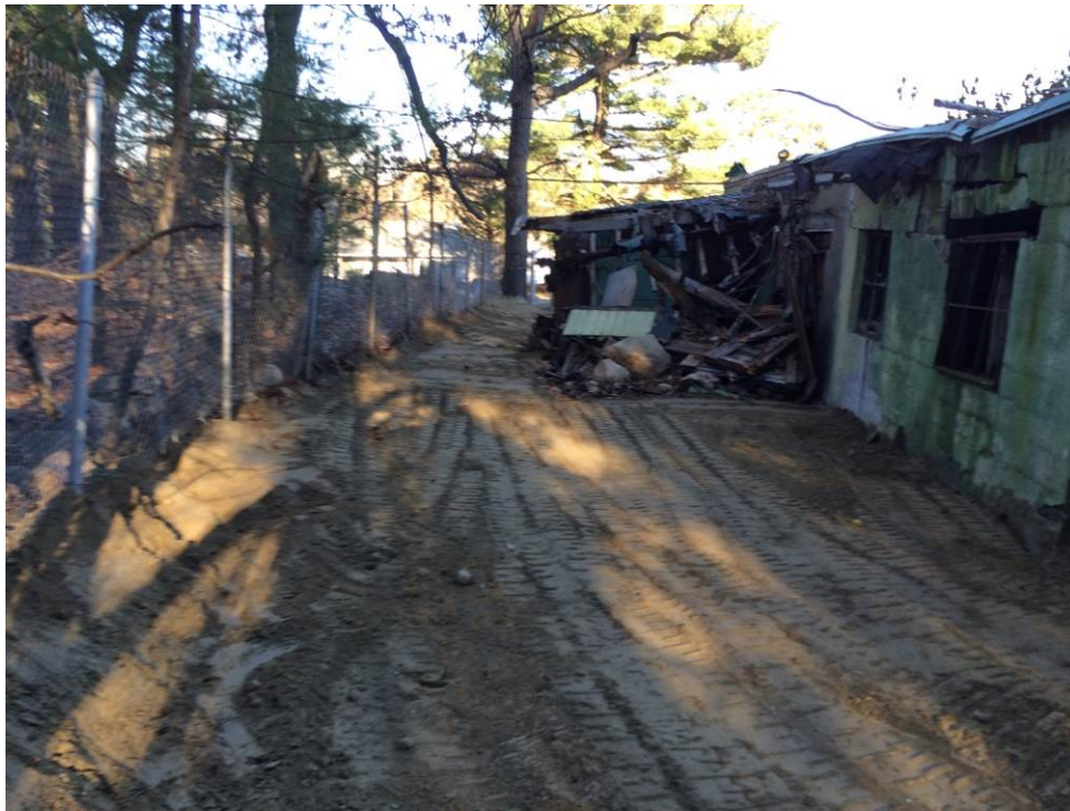
SCENE: View of final site conditions west of the lab building. Photograph taken facing north.
