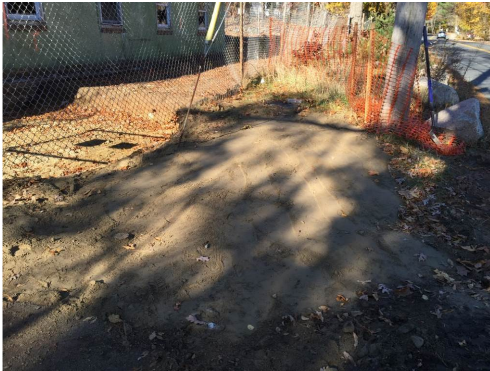
SCENE: View of the repaired water service line after backfilling and compaction activities. Photograph taken northwest.
