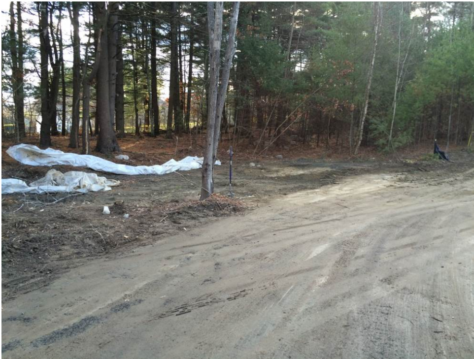
SCENE: View of the former location of RCRA drum carcass pile following load-out. Photograph taken south.
